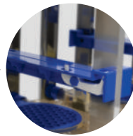
Incorrect Fitting/ No Cage
